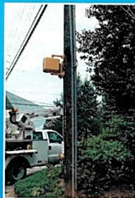
Electric & Existing Pole
