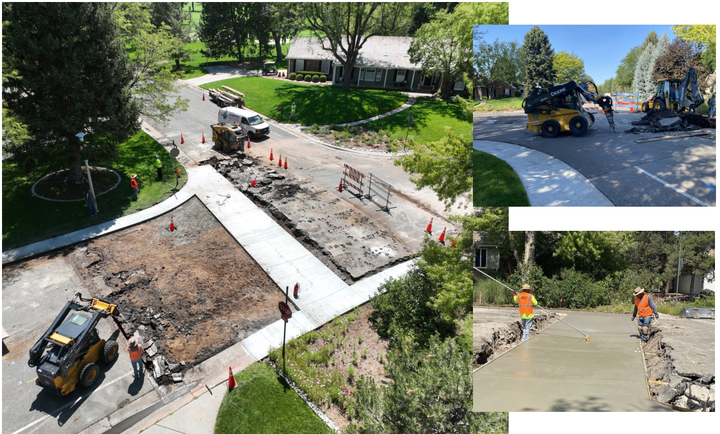
As of Aug. 9, the new concrete pans were in place at the intersection of Niblick and Club Lanes. The work is part of the annual town-wide paving project.
