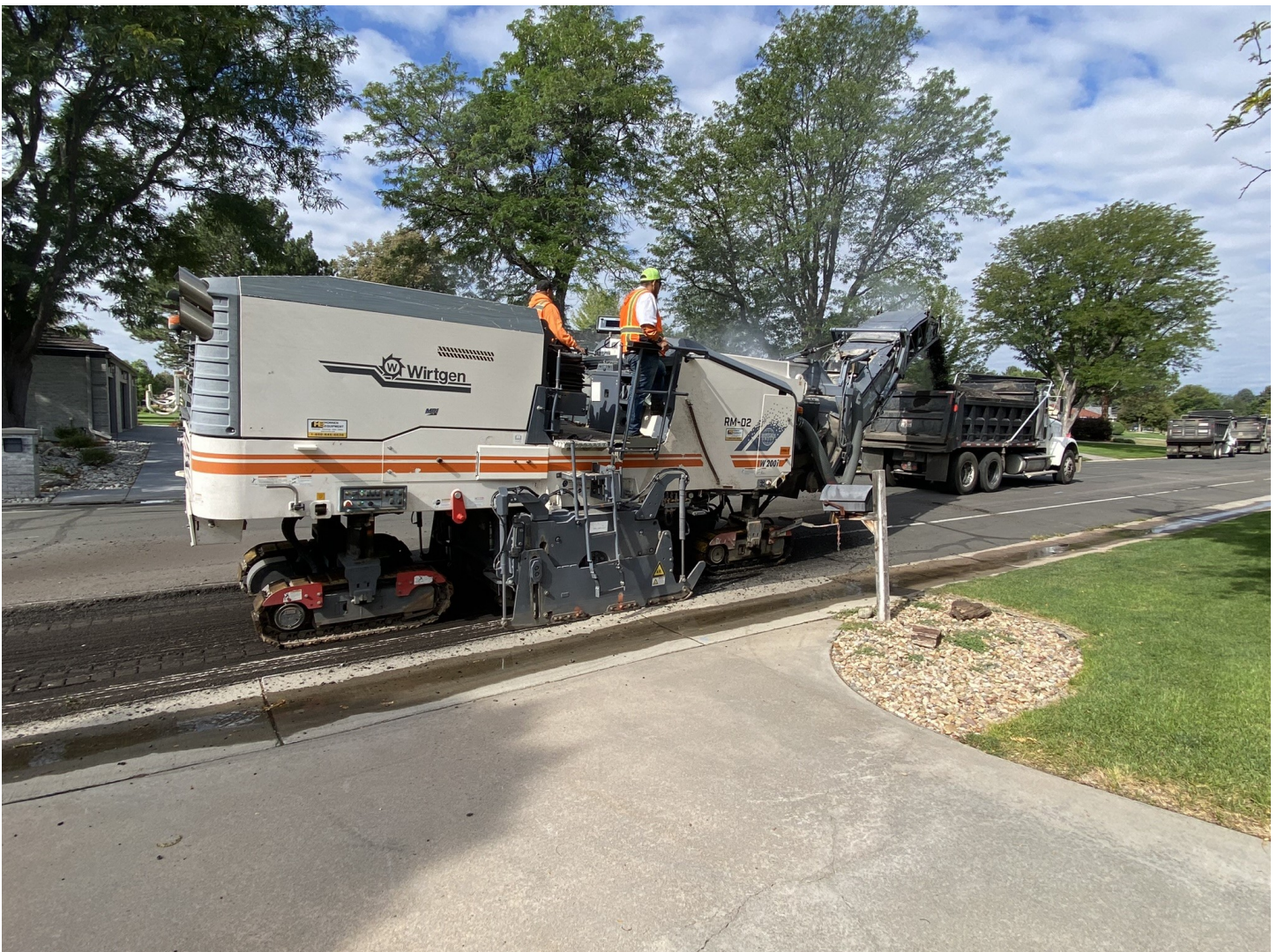
The milling machine removed the top 2" of asphalt before paving the streets where Denver Water replaced the water main.
