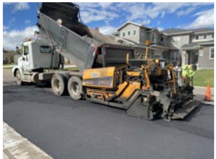
Above: Repairing sinking asphalt caused by saturated clay subgrade on Latigo Place.
